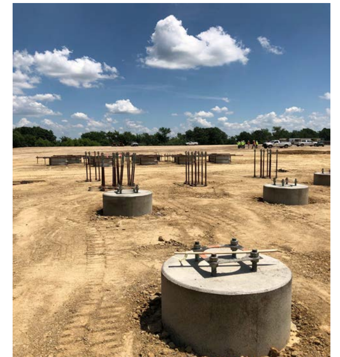
Newly poured foundations are installed at the Zachary Substation in Adair County.
