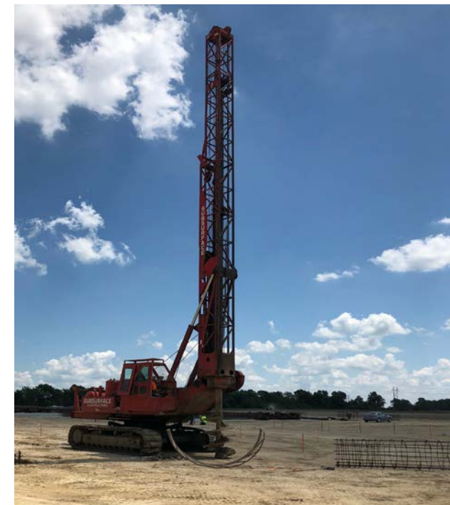
Before concrete can be poured, a drill rig creates the holes needed for Zachary Substation's foundations.
